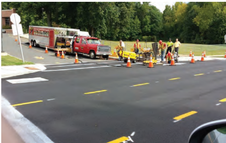
John Bossi, Mike Perry and a Plainville Police Officer oversee the work being done by the company installing decorative sidewalks on Northwest Drive in front of the Middle and Tofflon Schools. Slow down, watch the bumps!
