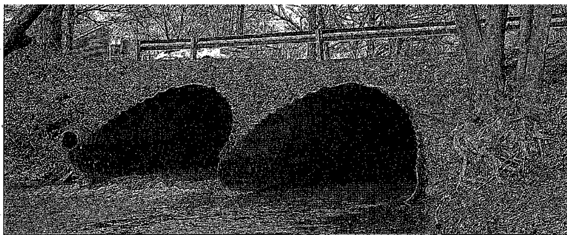
The Tomlinson Avenue bridge in Plainville, which is finally being replaced with work starting today.
